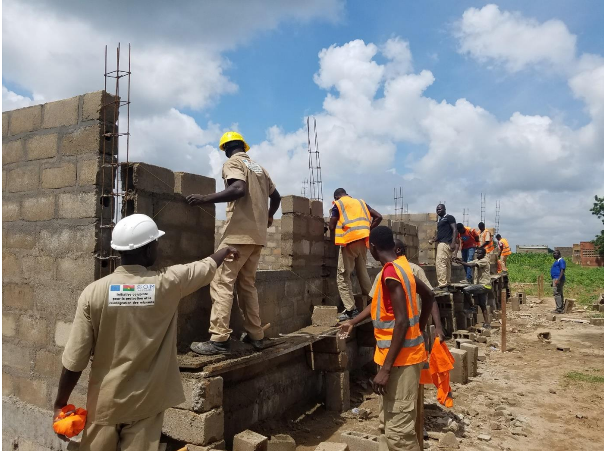
Figure 3: Returnees and community members on training site to rehabilitate community facilities. Photo: IOM/Judicael Lompo
